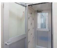
Air shower for eliminating dust
